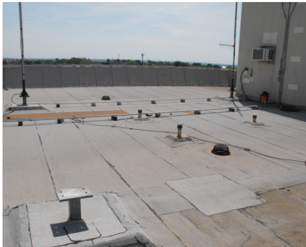
Left antenna is 146.805 & Right antenna is 444.95. New mounts for the masts of these two antennas
